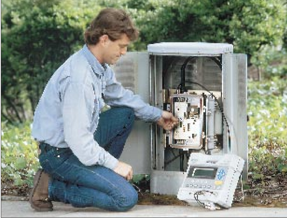
Return path alignment using the HP CaLan Sweep/Ingress Analyzer.
